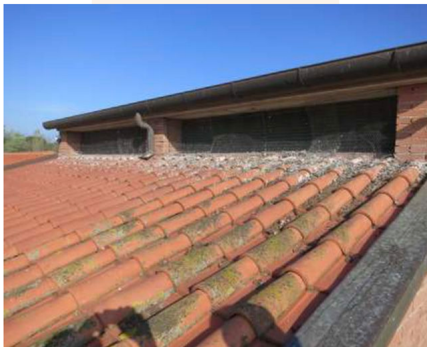
Figure 1. South roof prior to cleaning and treatment.
